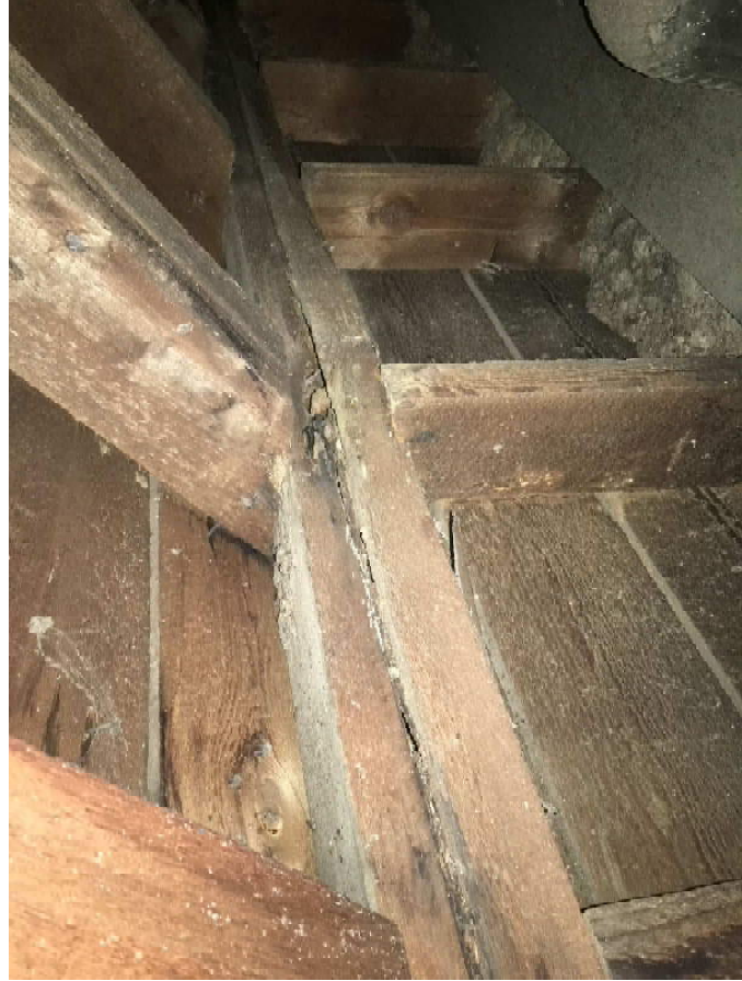
PHOTO 7: ROT AT TOP PLATE
