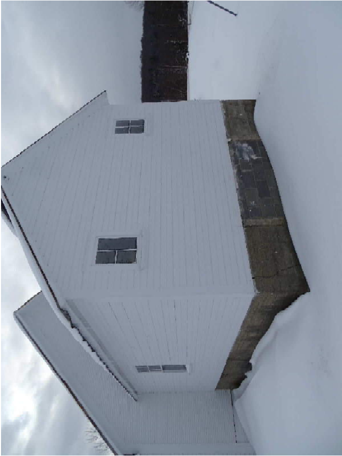
PHOTO 9: CRACKING IN NORTH ADDITION FOUNDATION
