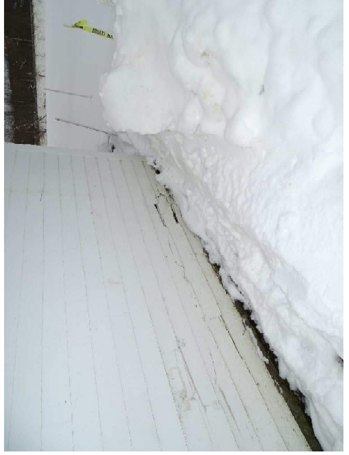
PHOTO 12: EAST ADDITION SIDING DAMAGE
