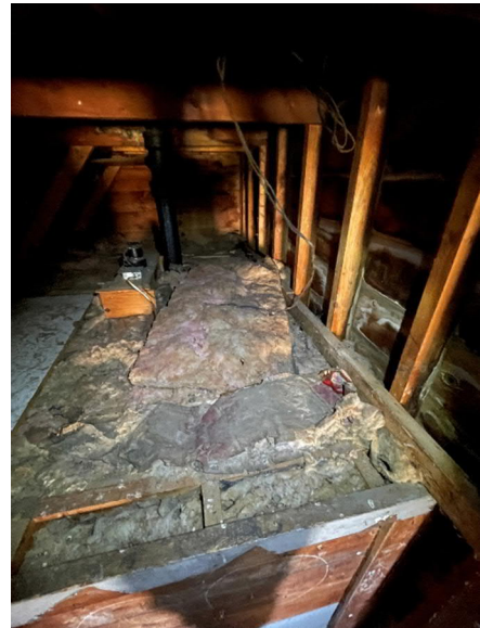
Figure 8 – Inadequate insulation over the bathroom
