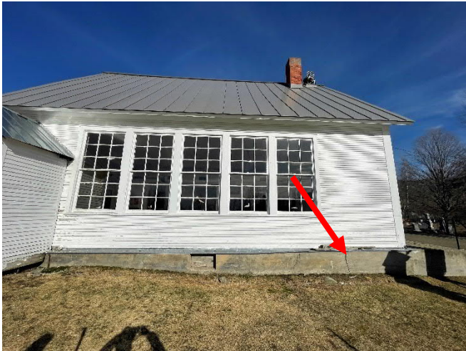
Figure 3 – Large crack in concrete foundation
