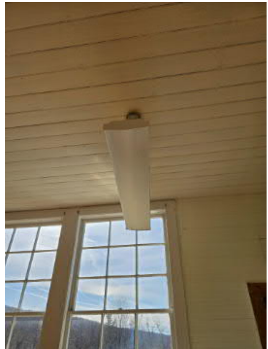
Figure 19 - Existing Interior Light Fixture with T8 Bulbs
