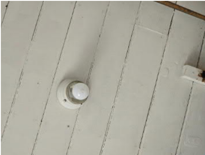
Figure 20 - Existing Interior Light Fixture with Incandescent Bulb
