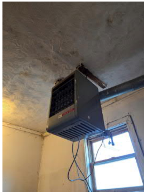
Figure 15 - Existing Unit Heater
