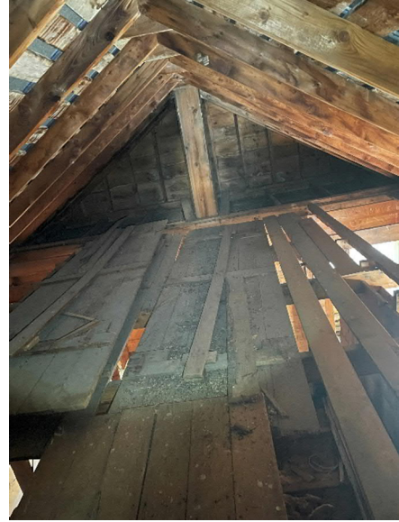
Figure 6 – Back attic with no defined air barrier
