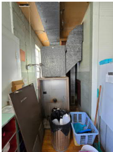
Figure 16 – Existing Ducted Furnace
