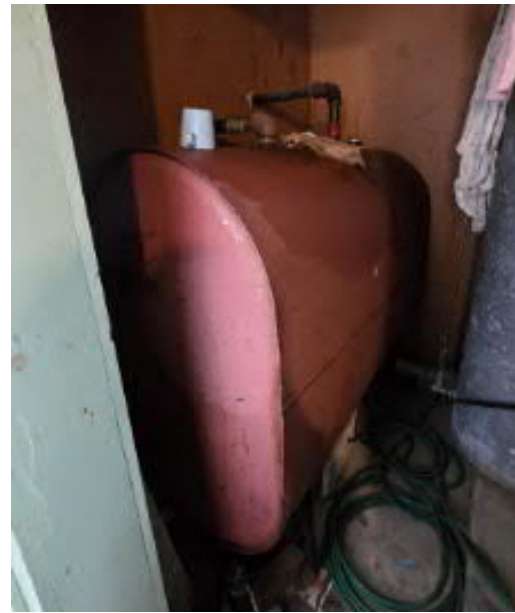
Figure 1 - Exterior Oil Storage Tank
